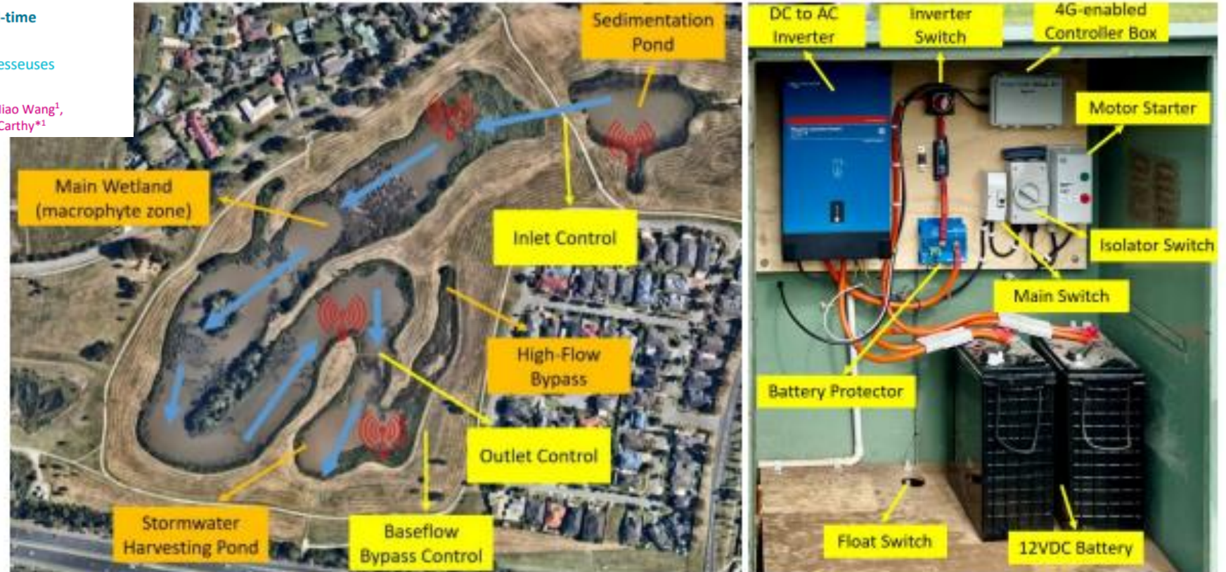
Figure 1: (a) Site Map of Troups Creek Wetland and the RTC control points. (b) Cabinet setup for the actuators installed at the control points. The actuator is placed behind the back of the cabinet.
